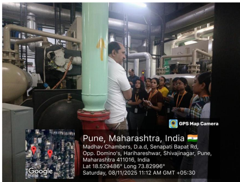
Figure 1- Students learning about chiller
